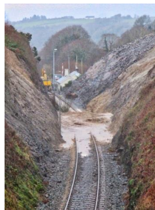
Plate 1 Landslide observed between Farranfore and Killarney on December 29 th , 2015 (photo credit: Iarnróid Éireann)
